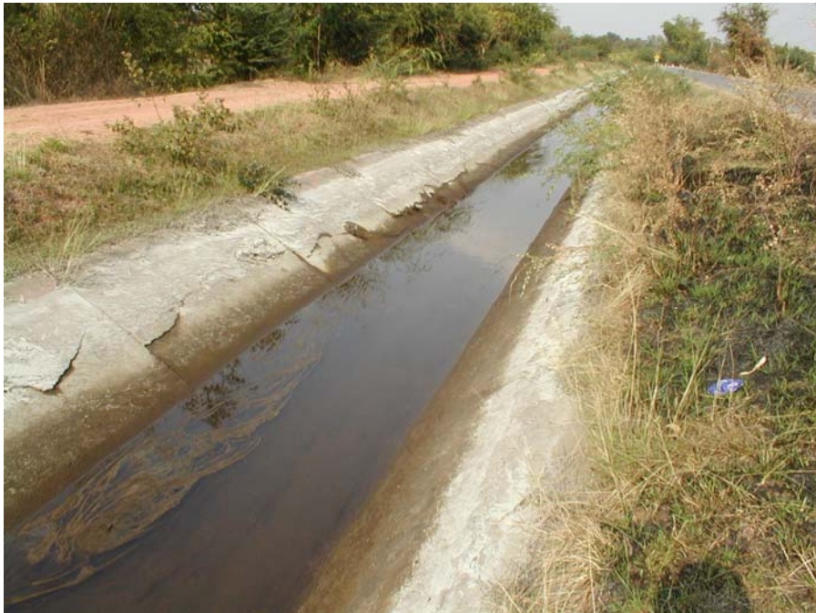
Figure 6.61 Salt crust on canal pavement in an irrigated area of the Sung Nern District, Nakhon Ratchasima Province.
