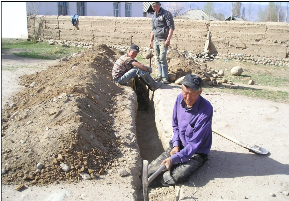
Figure 25: Villagers digging a trench for a private connection to the subsurface pipeline in Kara-Suu (Photo: Topbaev, April 2011).
