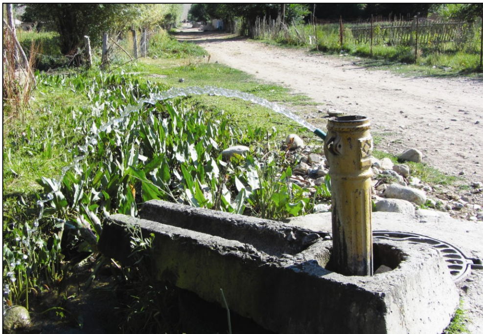
Figure 24: 'Working' standpipe in Kara-Suu (Photo: Topbaev, August 2012).
