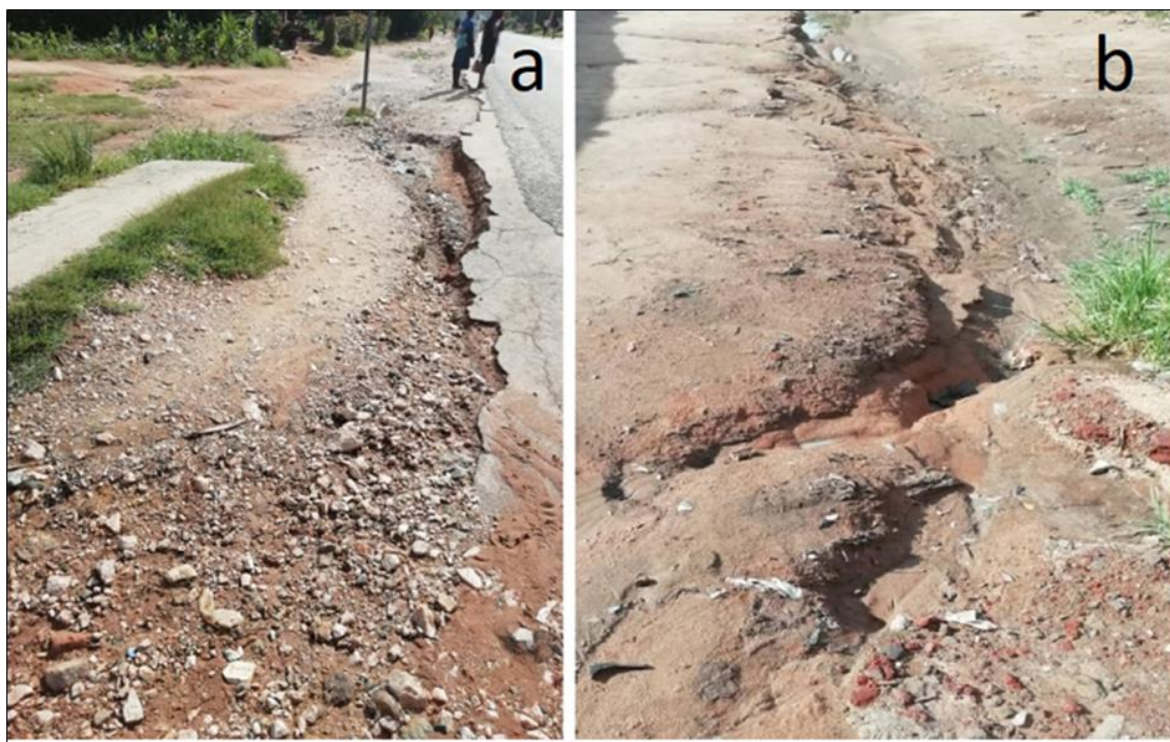
Figure 5.6 The extent of soil erosion observed in Epworth district. The extent of soil erosion observed in Epworth district. (a) paved roadside erosion feature; (b) erosion occurring in an unpaved road.
