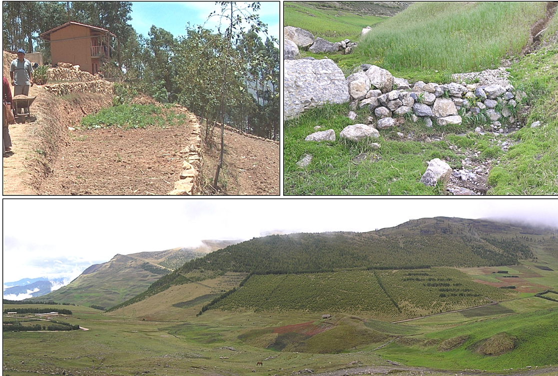
Figure 6–4: Measures of soil and water conservation in the region of Cajamarca. Upper left: Terraces at the demonstration site “Parcela Pablo Sanchez,” west of the city of Cajamarca (Photo: Schulte 2006). Upper right: Check dam in Choromayo, a headwater area of the Ronquillo basin (Photo: Krois 2009). Lower panel: Afforestation area in the Jalca orobiome, north-west of the city of Cajamarca (Photo: Krois 2009).
