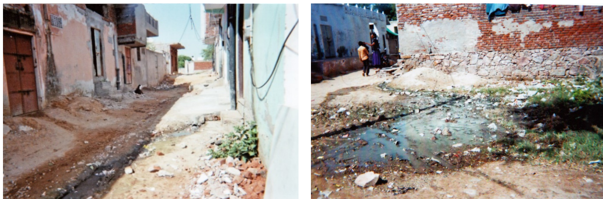
Fig. 49: Two examples of the photos taken by the women community leader from NKT: typical unpaved street in NKT with missing canalization for grey water (left side) and resulting water-logging (right side). September 2015, Jaipur.
