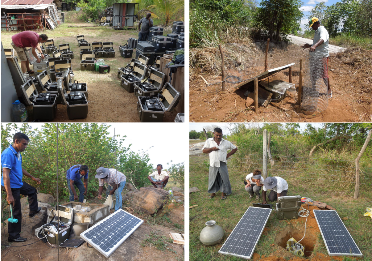
Figure II.2: Deployment of seismic stations (SL19, SL15, SL23) and preparation for shipping after deinstallation of the temporary network (top, left). Solar panels were installed at half of the stations, which was the preferred source of energy.
