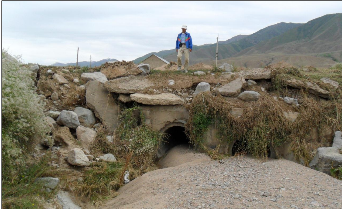
Figure 30: Culvert of Topon-Aryk clogged with sediment (Photo: Topbaev, 2010).
