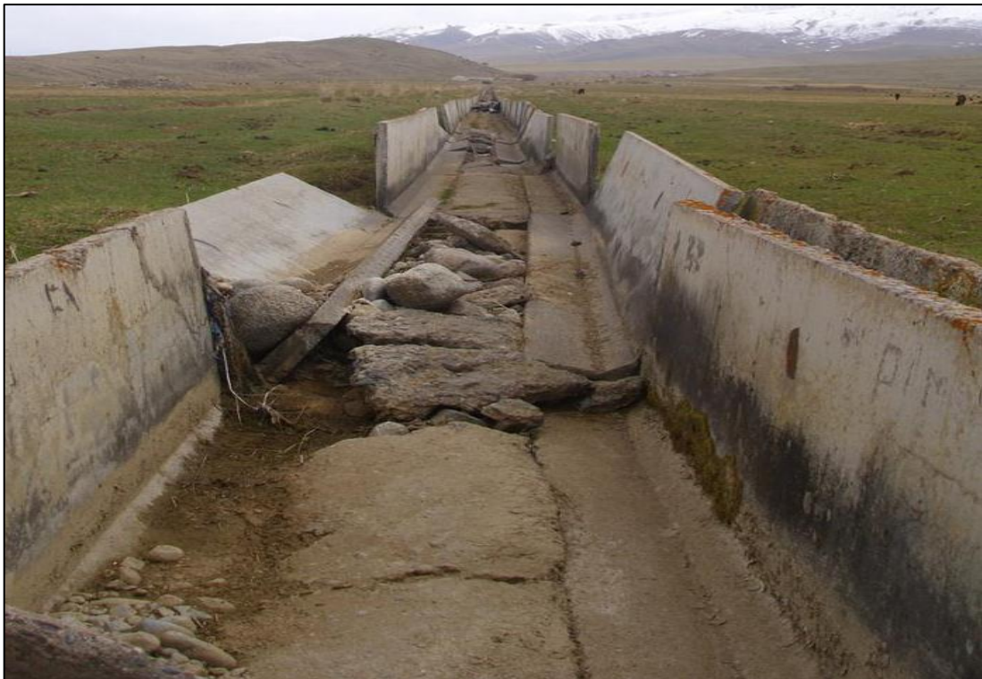
Figure 33: Poorly maintained on-farm canal in the vicinity of Kara-Suu (Photo: Ebermann, 2011).
