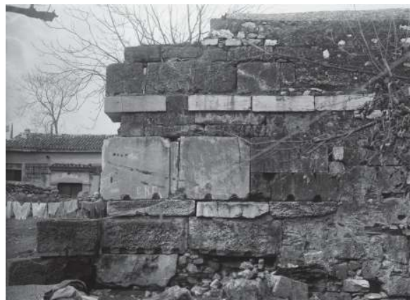
Fig. 6 The so-called Post-Herulian Wall adjoining the dismantled section near Ag. Dimitrios Katiphoris.
