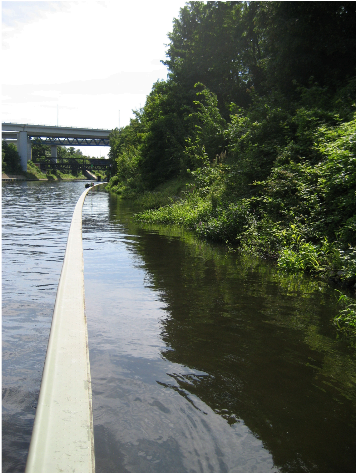
Figure I.3: Rehabilitation site built in 2008 at the Teltow Canal, Berlin, Germany. The image was taken on the 6 th of July 2009, facing upstream from N 52° 27' 29.9", E 13° 24' 29.7".
