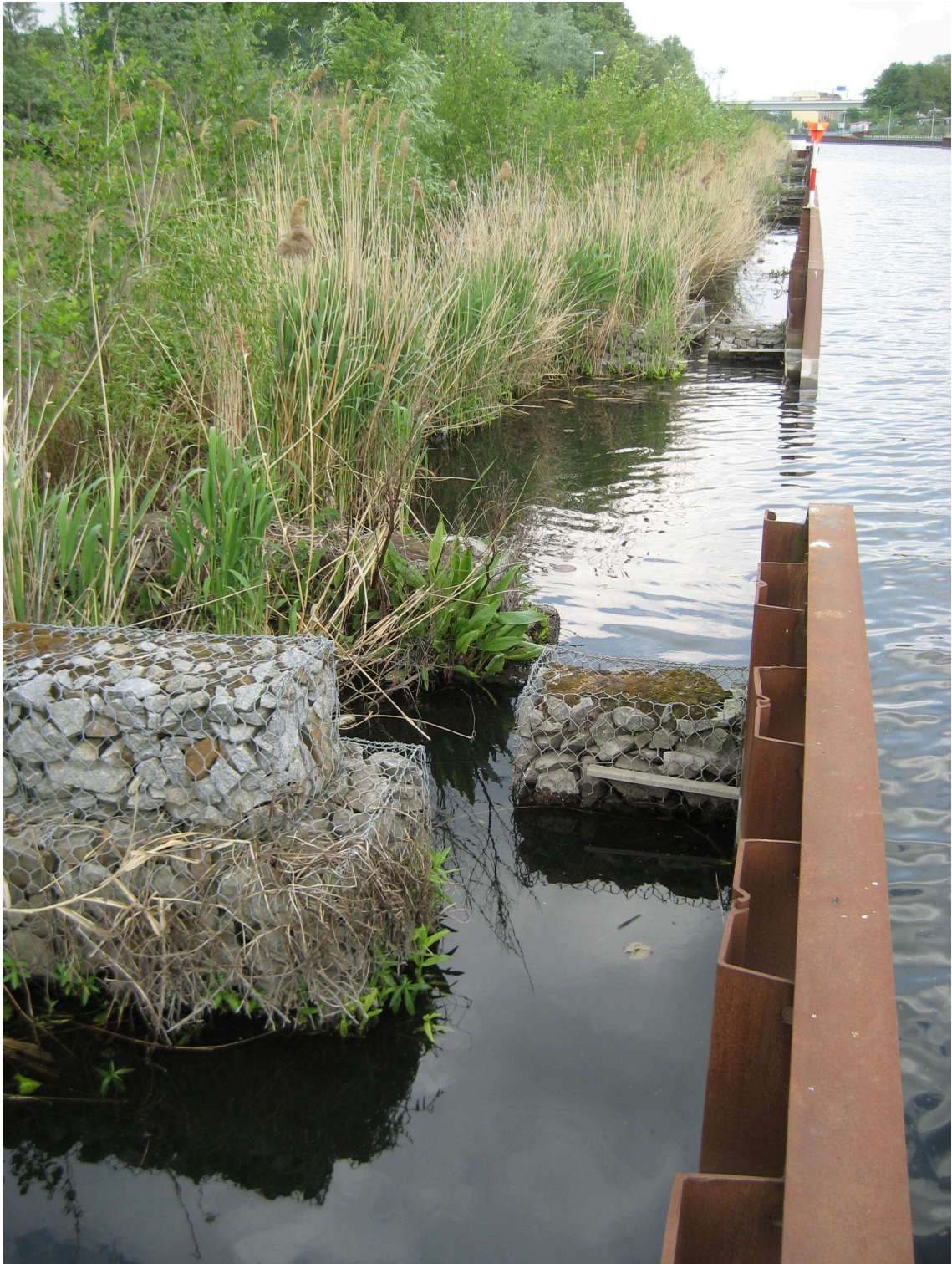
Figure 2.9: Structure of the gabions at one representative opening of the rehabilitation structure at the River Spree on the 7 th of May 2009.
