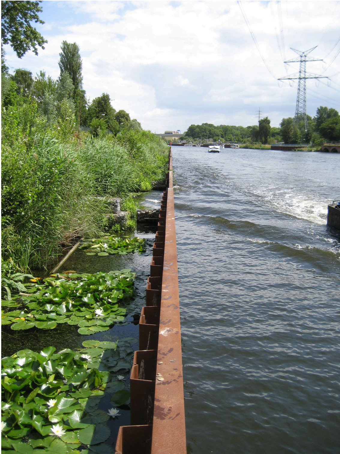
Figure I.2: Rehabilitation site built in 2004 at the urban River Spree, Berlin, Germany. The image was taken on the 6 th of July 2009, facing upstream from N 52° 31' 45.6", E 13° 16' 18.5".
