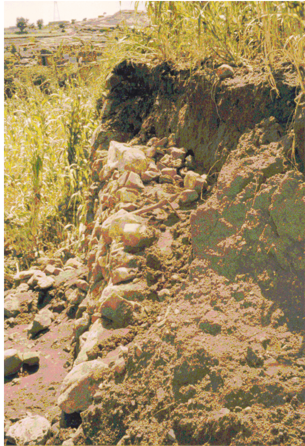
Photograph 4.3 Eroded terrace under construction (lower part is already rebuilt). This Terrace broke down after a series of heavy rainfalls. It is clearly to recognise that the wall leans against the soil. A thick root was growing against the wall from inside which destabilised the terrace wall. The total length of the terrace damage increased within 3 – 5 days from 3 m to approximately 12 m because the farmer decided to wait with the repair of the terrace.
