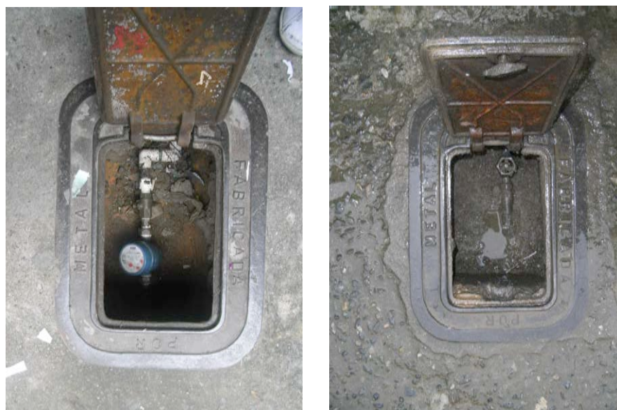
Figure 28 Removal of a water meter by contractors of EPM to avoid illegal reconnections
