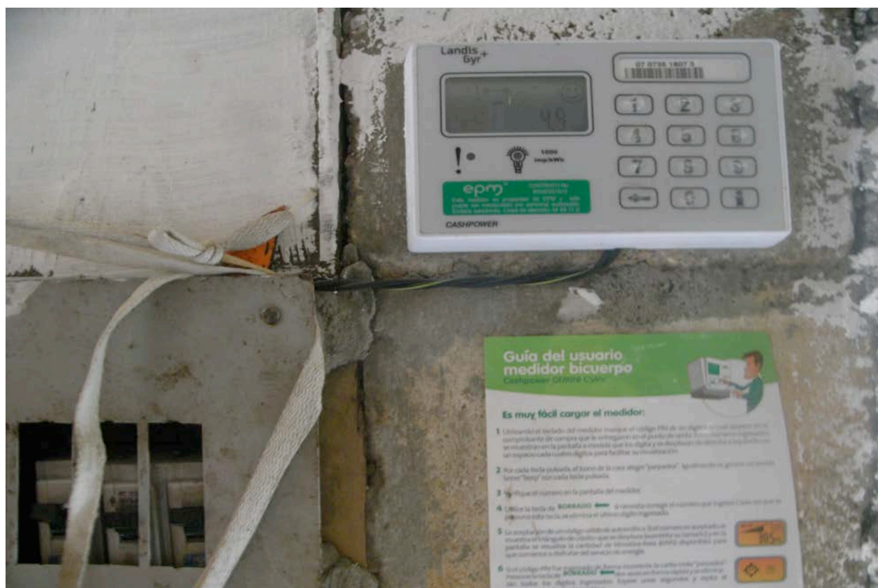
Figure 25 Prepaid electricity meter installed in a household located in the barrio El Limonar
