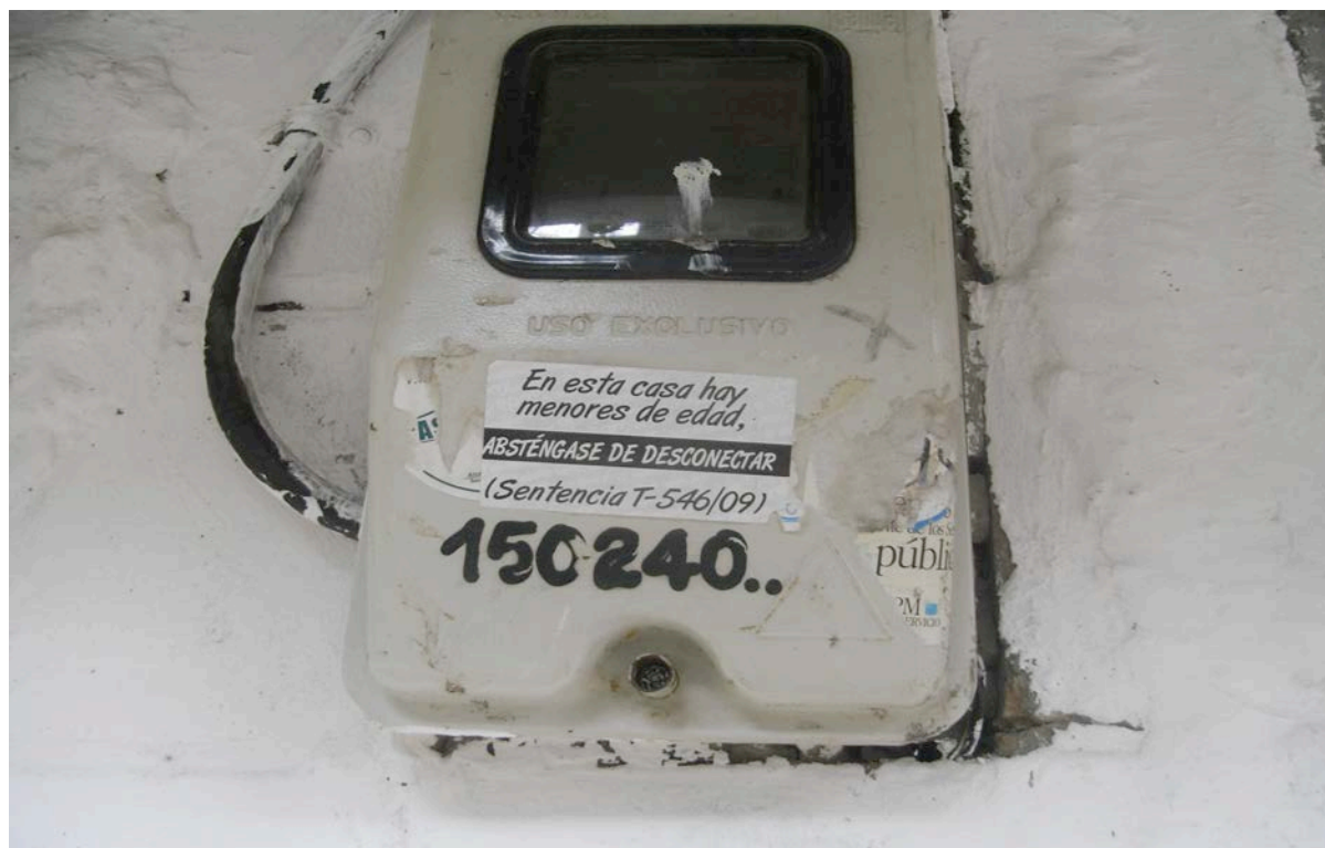
Figure 26 Awareness campaign placed in the electricity meter located in the façade of a low-income household to prevent disconnection
