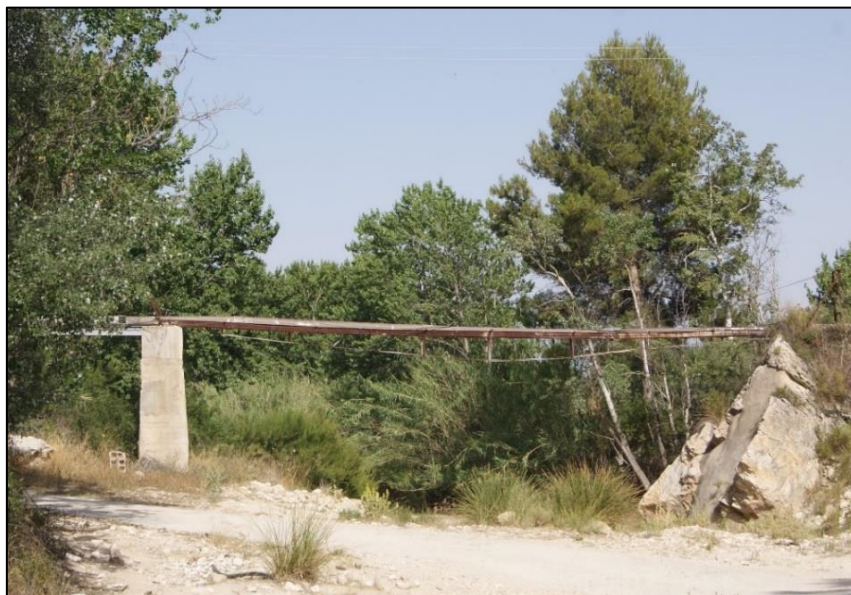
Fig. 7: Aqueduct bridging the riverbed of the Río Claro in the vicinity of the Cortijo Corneros (for its location, see Fig. 10).
