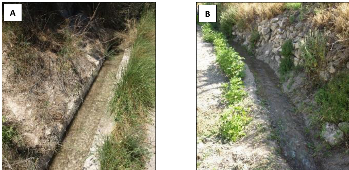
Fig. 2: Irrigation channels in the Vega of Vélez Blanco. A: Modern concrete irrigation channel. B: Traditional earthen channel on an agricultural terrace within the Vega.
