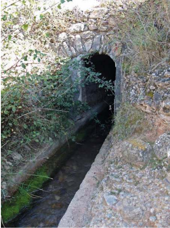
Fig. 9 Cimbra at Bulbunte, Zaragoza, running beneath the stream bed of the River Huecha.
