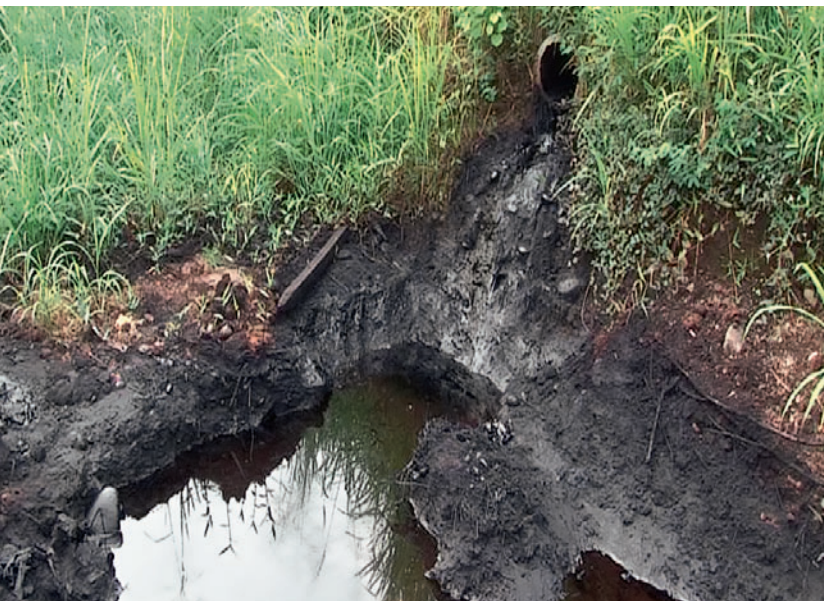
Defekte Ölpipeline in Ecuador | Damaged oil pipeline in Ecuador
