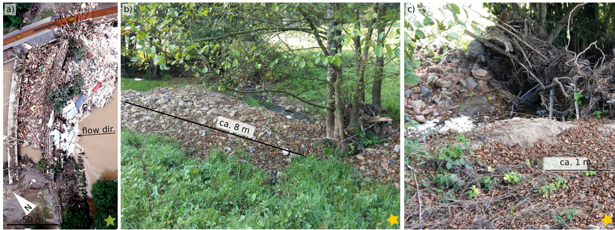
Figure 5. Effects of large woody debris. For locations on wider map see stars in Fig. 1. Pair of clogged bridges near Altenahr, bypassed along the left and right bank. Note the bipartition of the collected debris with woody material caught by the downstream road bridge and anthropogenic debris collected later by the upstream railway bridge. Note two remaining standing trees in the river depicting the width of the Ahr River before the flood. Aerial image by BBK-DLR (2022). (b) Huhnenbach near Aremberg about 2 km from its source (see Fig. 1). Note clogging by woody debris at riparian trees and the resulting ejection of coarse bed material out of the channel. (c) Another clogging of the Huhnenbach some 20 m upstream of panel (b) , with both ejected coarse debris and deposition of fine sediments in front of the obstacle.
